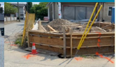
Does not meet standards: Truncation is not 3x3 metres
