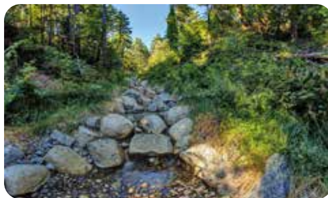
Stabilization project on steep slopes along John Matthews Creek. Photo Credit: Burnaby Now
