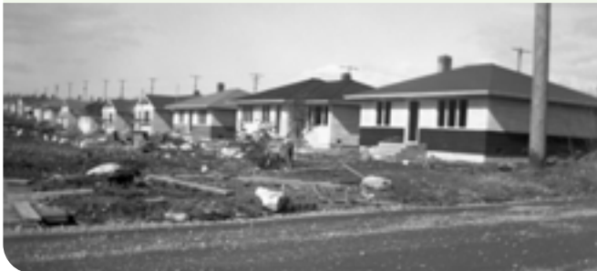
Suburban houses under construction in Willingdon Heights in 1947. City of Burnaby Archives 010-032
